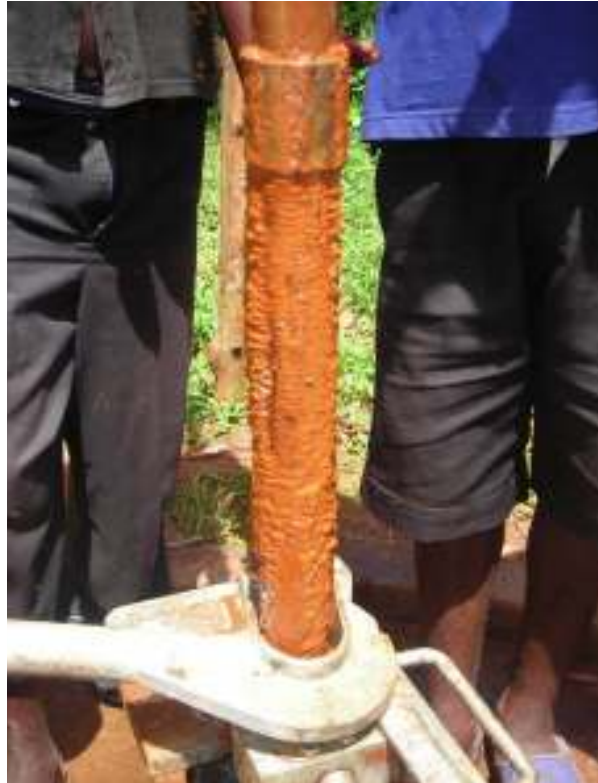
Figure 1.2 Orange slime found on galvanized iron riser pipes extracted from the well in Bulegete (photograph by author)
