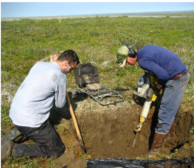
Figure 89. Digging in permafrost in the tundra, using a jackhammer. Photo by Nick Bonzey, through Creative Commons.
