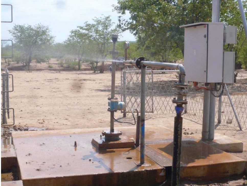
WW29047 with leak (1/19/2014)
