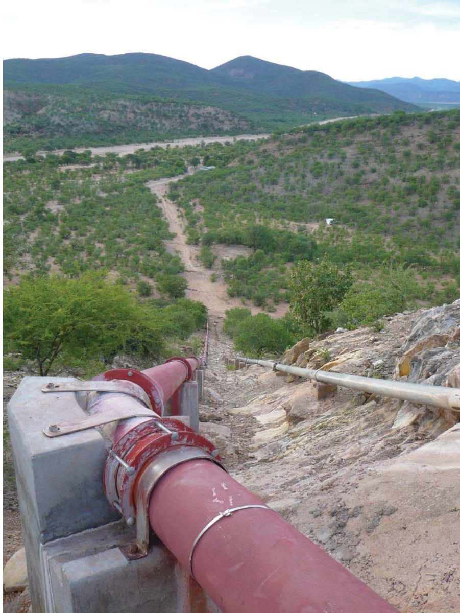
Pipeline from NamWater Plant to storage tanks. Note old pipe situated parallel to current pipe.
