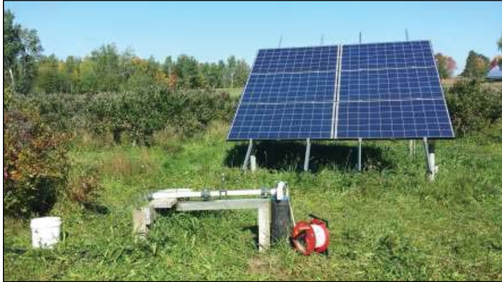
Figure 10: Solar pumping set-up at Gierke Blueberry Farm, September 2014
