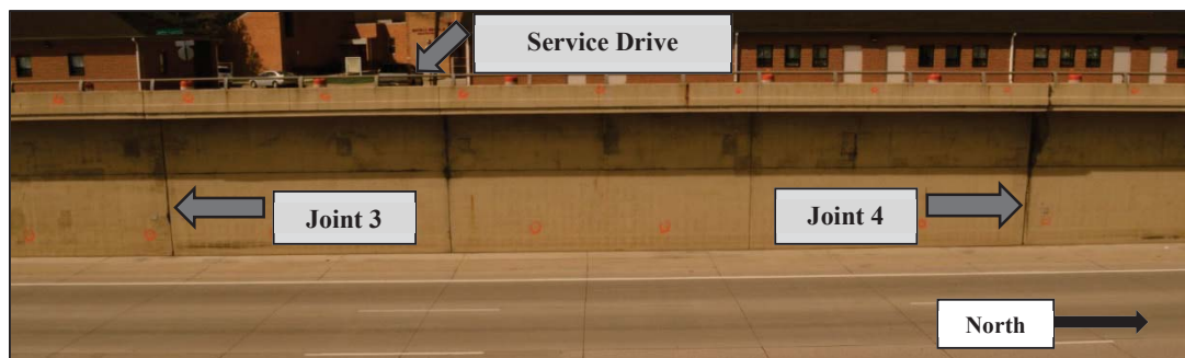
Figure 1-4 Section of retaining wall which experienced the most movement at the Meyers site on M-10 highway between Joint 3 and Joint 4.
