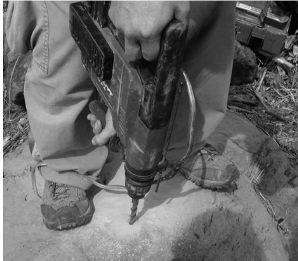
Drilling into rock. Using a hammer drill we perforate rock to install our benchmarks pins. Photo by author.
