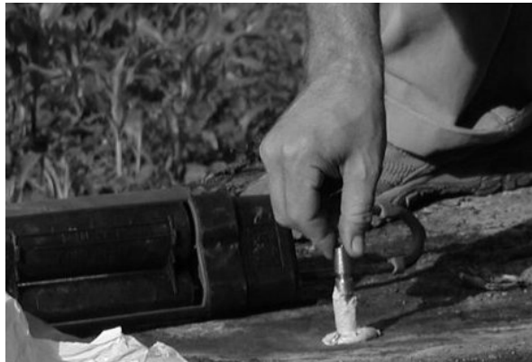
Anchoring the benchmark. Using Hilti epoxy we anchored the benchmark in the rock. Setting the pin flush with the surface discourages theft and vandalism. Photo by author.
