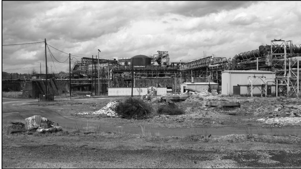
Figure 5.8 Copperhill smelter and acid plant as it looked in April 2008 after years of successive demolition and removal projects. (Source: author)
