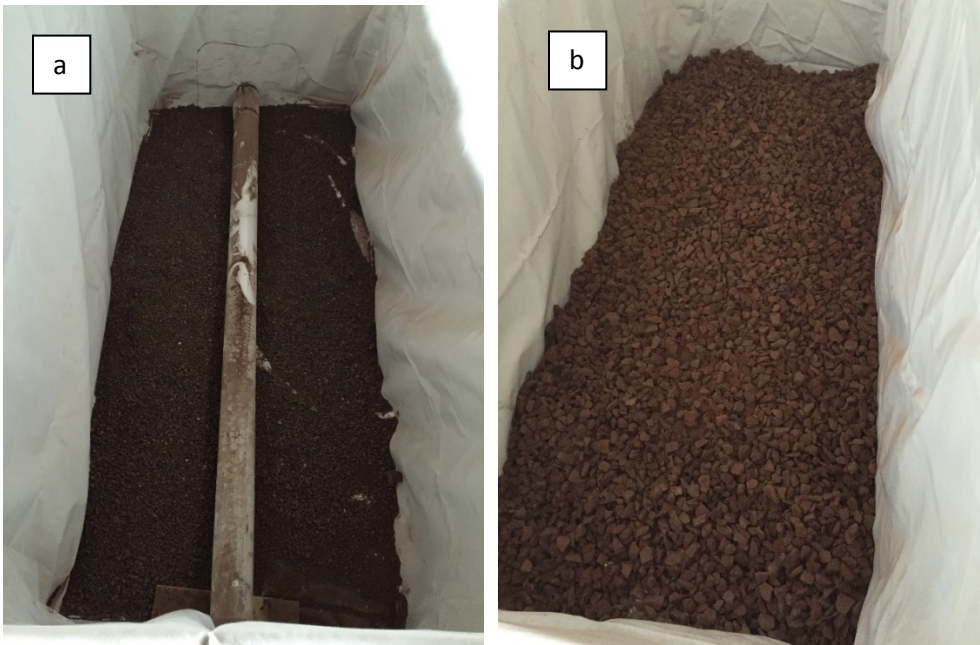
Figure 2.4. To construct the drainage system, first (a) Small gravel was added below the drainage pipe, followed by (b) size 6A gravel were added for drainage.
