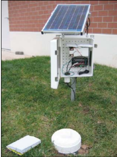
Figure 11. Power and communication equipment set-up using the CR206 datalogger by Campbell Scientific, Inc. from Logan, Utah. Photo taken in November 2006, (Copyright 2006, Wetland Studies and Solutions, Inc.).
