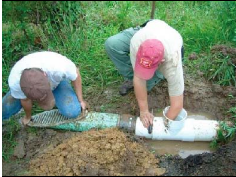
Figure 9. Installation of fabricated fitting and stilling well at monitoring location DP4 towards the north end of the site. Photo taken September 27, 2006, (Copyright 2006, Wetland Studies and Solutions, Inc.).
