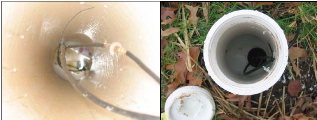
Figure 10. Installation of Model 8000 level sensor into stilling well (two locations pictured here). Sensor is mounted on semi-flexible cable extending to the top access point of the PVC design. Photos taken in November 2006, (Copyright 2006, Wetland Studies and Solutions, Inc.).
