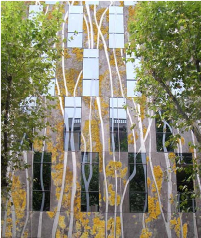
Figure 37. Simulation of a vegetated facade at the Ako-Suites Aparthotel in Barcelona, Spain. Photo from Escofet 1886, S.A., courtesy of Sandra Manso Blanco.
