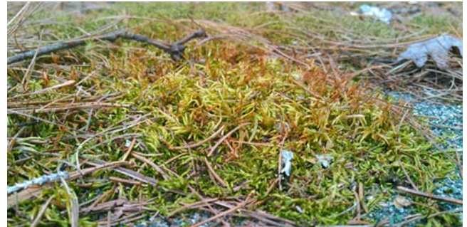
Figure 104. Mosses growing on an asphalt tile roof. Photo by Annie Martin, with permission.
