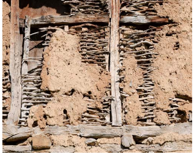
Figure 12. Wattle and daub construction, with sometimes uses mosses in the mud daub. Photo by Pany Goff, through Creative Commons.
