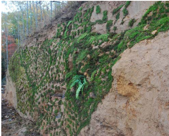
Figure 63. A completed portion of the clay wall. Photo courtesy of Annie Martin.
