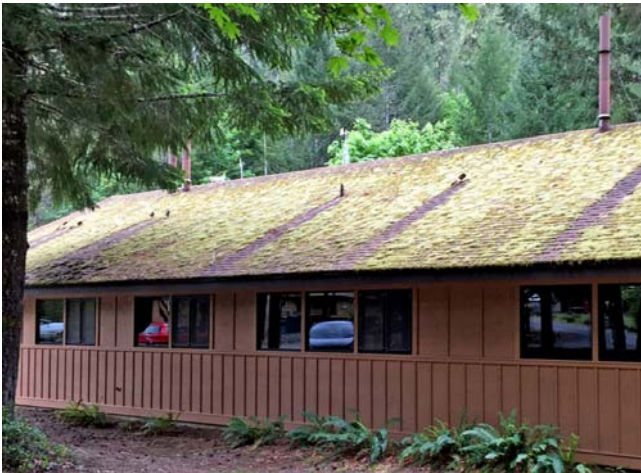
Figure 77. Moss roof and zinc plates that prevented moss growth down-roof. Photo by David Wagner, with permission.
