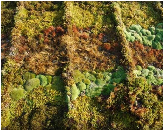
Figure 99. Moss roofing completed showing variety of colors and patterns. Photo by Annie Martin, with permission.
