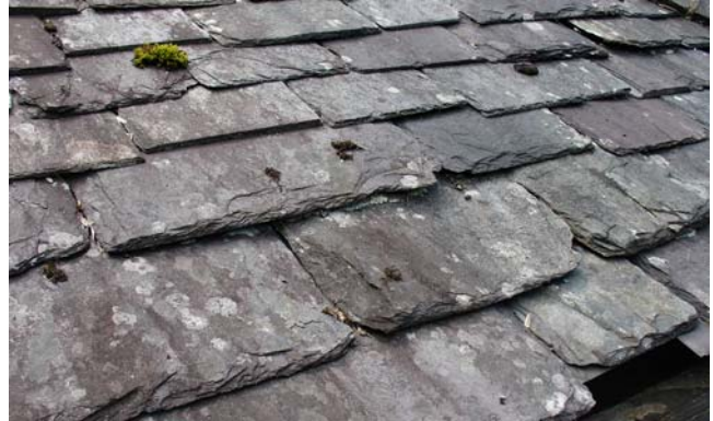
Figure 23. St. Fagans Tannery, Wales, slate roof with mosses that have arrived after construction, along with many crustose lichens. It appears that this one might be laid on a bed of mosses beneath the slate. Photo by Zureks, through Creative Commons.
