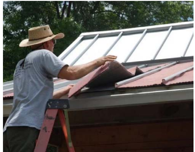
Figure 96. Laying the substrate on the metal roof. Photo by Annie Martin, with permission.
