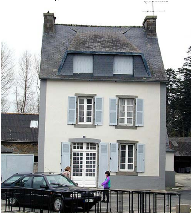
Figure 137. This house in Bretagne has mosses invading the roof. Photo by Michael Lüth, with permission.
