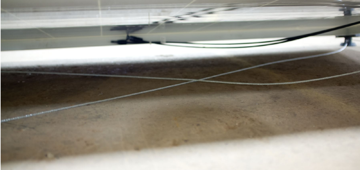
Figure 1: Steel wires crossing under the PV module in the X-wire system.
